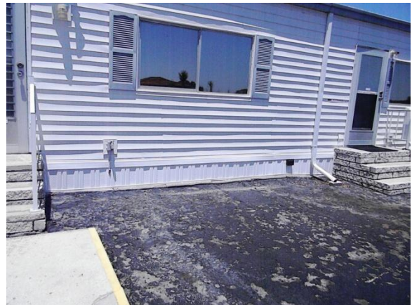
Photo by Randy Doell Under-pinning completed on the East side of the corporate office.
